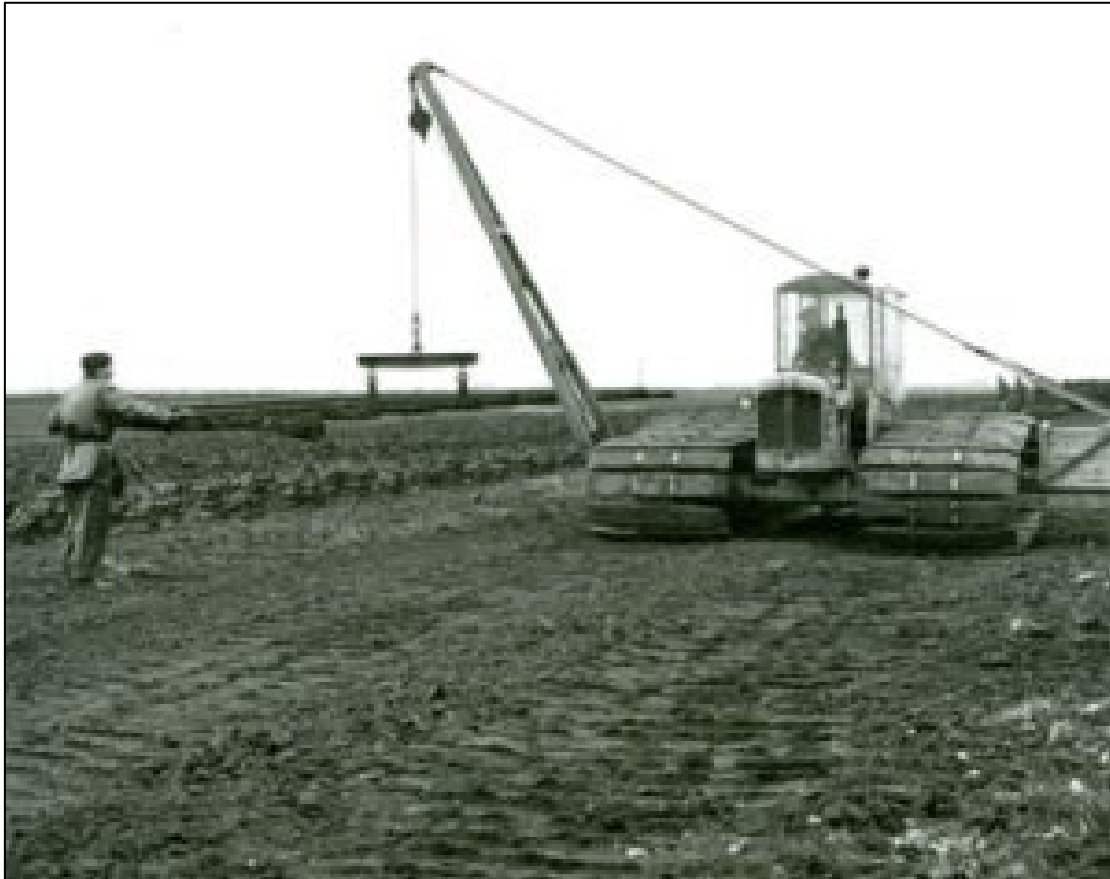
Plate 4-38: Rail Moving Attachment to lift and lay temporary railway track, along Sod Peat ricks and milled peat piles. (Source: https://www.bordnamonalivinghistory.ie/equipment-detail/rail-moving-attachment/ )
